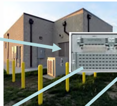
Airport Lighting Vault (secure)
